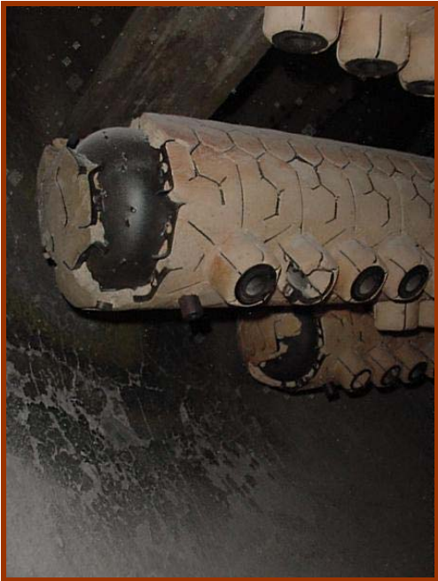
Fig. 07 - S-bar weld failure on Air Grid Arms
