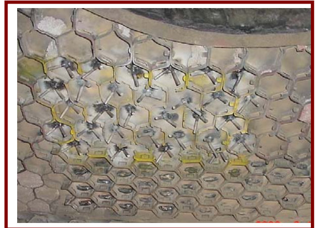
Fig. 02 Before - Hexmesh with addition of single point Vee anchors on Cyclone Roof.
